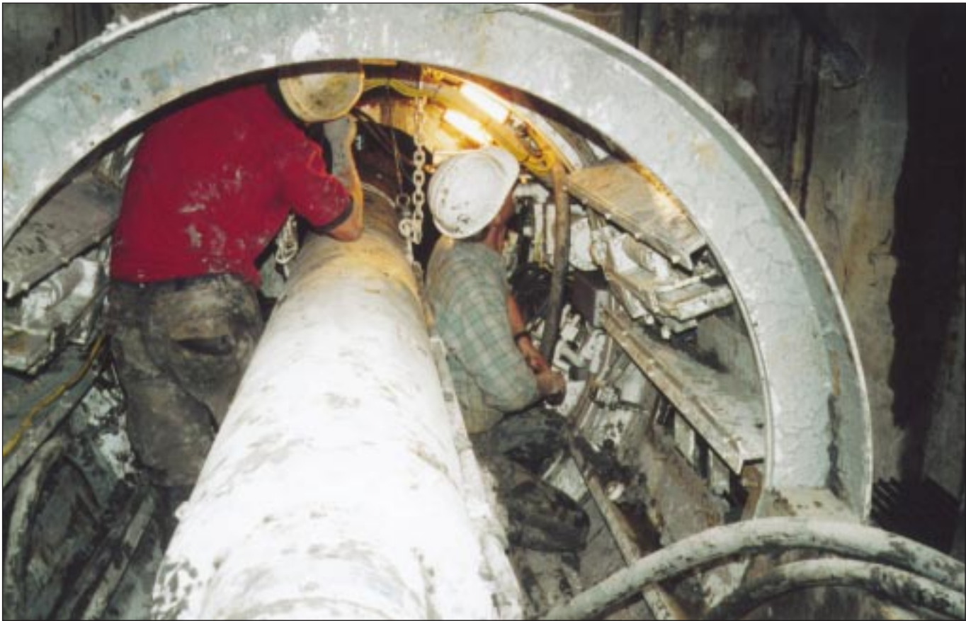
Photograph Above. Setting up for the tunnel drive. The launch of the TBM is unbelievably fast. From lowering in the shield to burying the first pipe a time of under 40 minutes was recorded by NATM.
