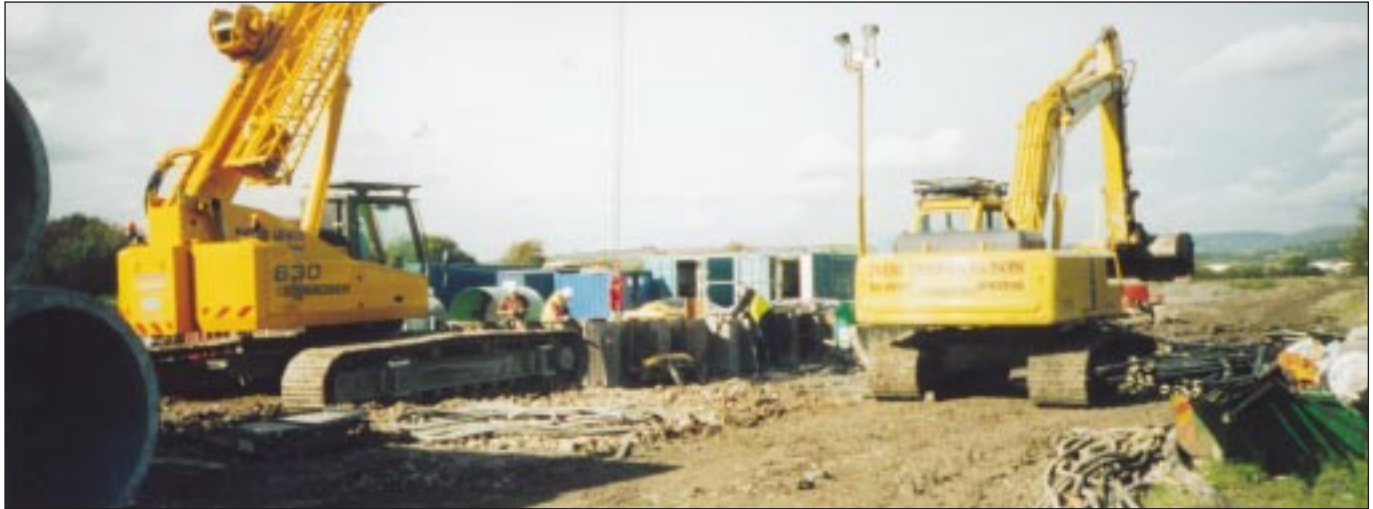
Photograph Above. 2 No. excavators serving the tunnelling operation. The TBM mined at such a speed that a specially adapted and much larger skip had to be manufactured by PL Manufacturing. A staggering 187 ft was driven in 1 No. 12 hour shift.
