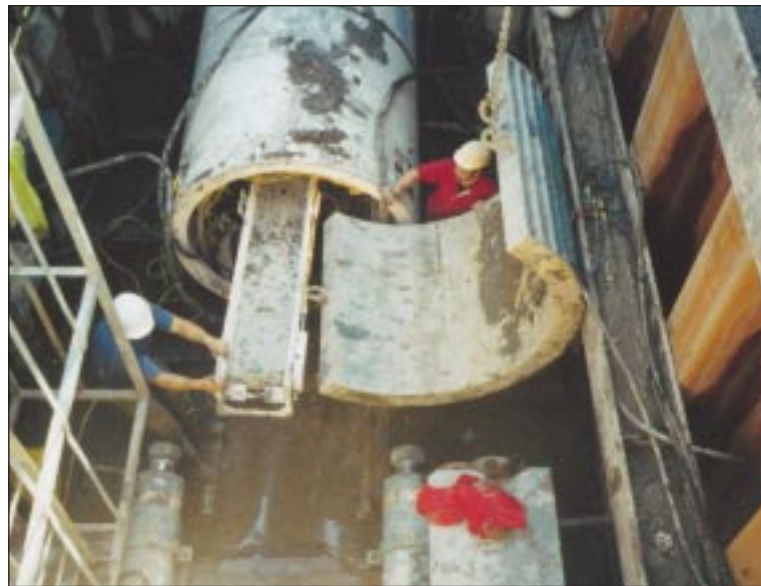
Photograph Above. Lowering down one of the half moon spacers and preparation of the first pipe to be jacked.
