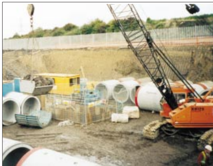
Photograph Above. B & W are handling the 2.5m long Hepworth pipes and removing the spoil from within the tunnel via a 30t track mounted Hitachi F125
