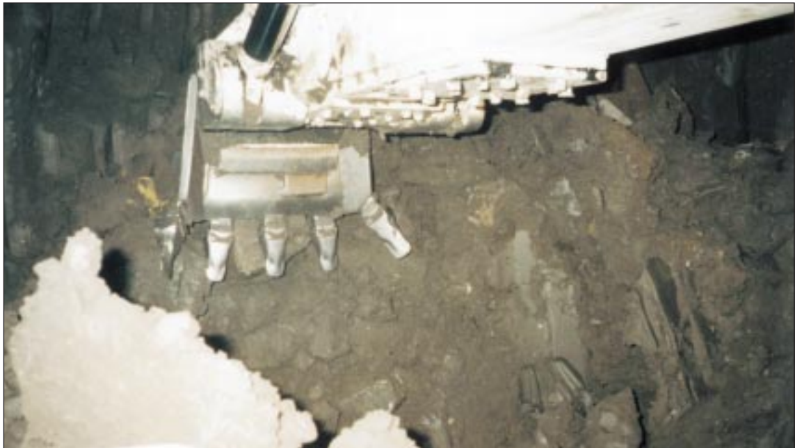
Photograph Above. The telescopic arm of the backacter is mounted from within a roof-mounted bearing, which operates off of a slew-ram within the centre of the shield and provides a 40-inch (1.01m) stroke.
