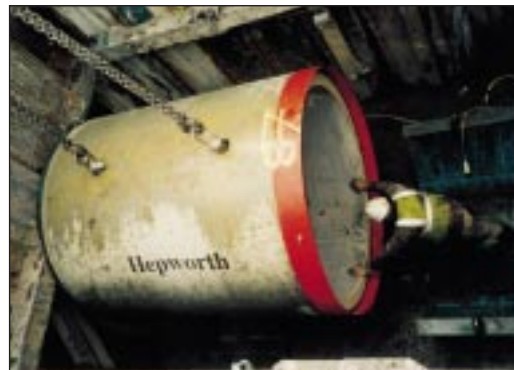
Photograph Above. Lowering the 2.5m long Hepworth jacking pipes down into the sheet and framed drive pit
