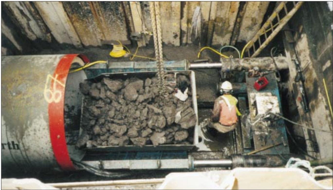
Photograph Above. Mucking out in the pit bottom. Director for B&W Tunnelling Steve Williams explained: "If this type of job was done by hand we would probably have to go 24 hour working producing a maximum drive of 4 no. pipes (2.5m long) in 24 hours. By going mechanical from start to finish we are averaging 5 no. pipes on a 12 hour shift basis."
